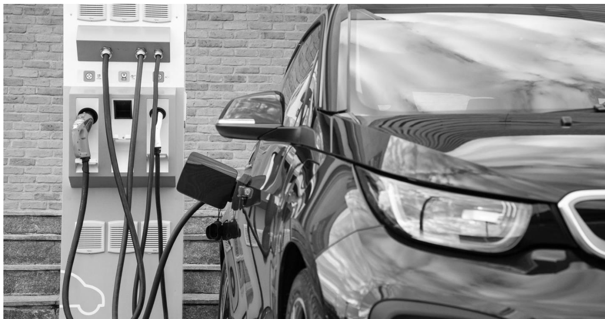
Figure 2. Photograph of a DC fast charging unit installed as part of the electric corridor Sao Paulo and Rio de Janeiro [47]
